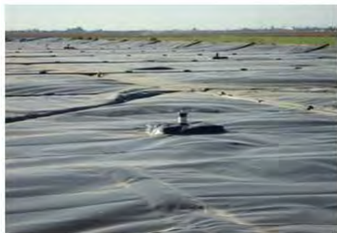
Covered Lagoon Digester
